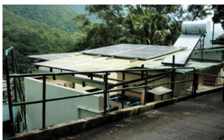
Photo-voltaic panels installed on the roof of the Veterinary Hospital.
