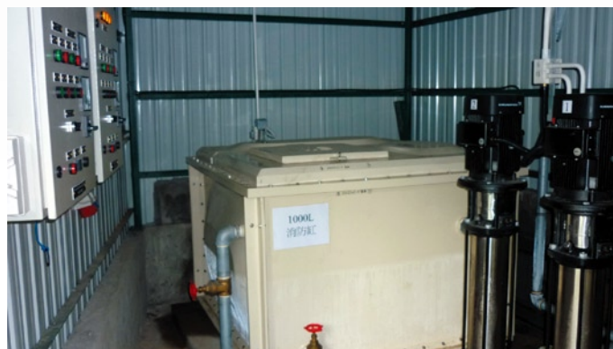
Interior view of the new Pumping Station for water supply from the Water Supplies Department.
