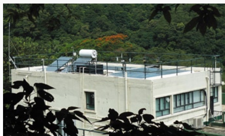
Photo-voltaic panels installed on the roof of the Conservation Building.
