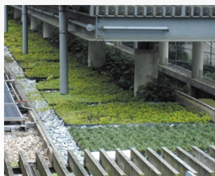
Sedum and Blue Grass were planted on the green roof at the Reception Building.
